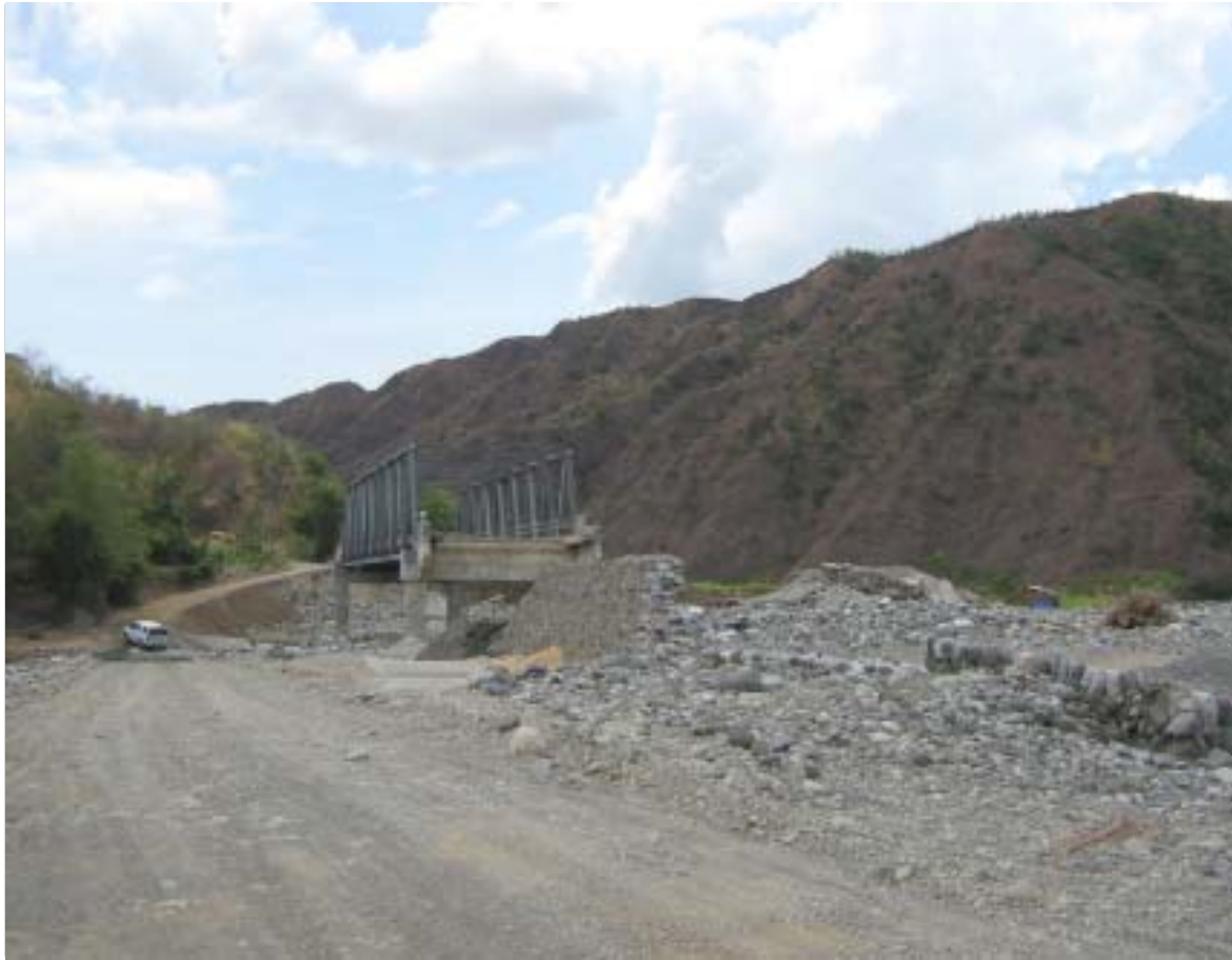
THE damaged Boao Bridge in Vintar, Ilocos Norte is set to be rehabilitated following the visit of Ilocos Norte Gov. Michael Keon in the said locality.
